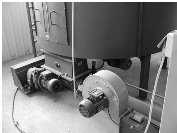
Slika 10. Pužni transporter za dobavu piljevine iz silosa u peć – problematično rješenje Figure 10 Conveyor worm for sawdust delivery from silo to power plant – problematic solution
